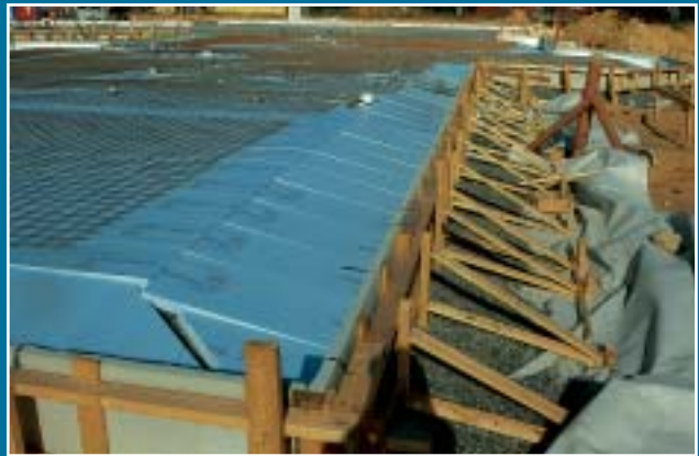
Elementary School near Stockholm, Sweden. Insulated stay-in-place slab edge forms (EPS coated with 1/2-inch high-strength concrete) and sub-slab insulation under monolithic FPSF. In Scandinavian countries, 2-inch thick insulation, either EPS or XPS, is widely used under concrete slabs to keep the concrete warm for thermal comfort.
