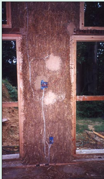
Wiring for the first floor (shown at right) was run along the surface of—or within—bales before stuccoing (above).
