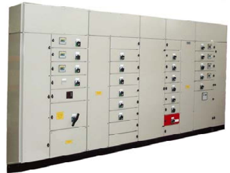
LV switchboard with multifunction meter on incoming lines and kilowatt-hour meters on selected outgoing circuits.
