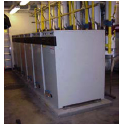
Modular boiler installation
