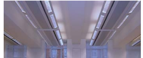
These chilled beams incorporate lighting as well as cooling
