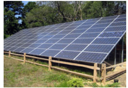
PV array, Wellfleet Wildlife Sanctuary, Massachusetts
