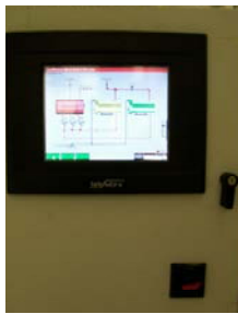
Energy management system
