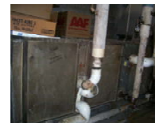
Flow balancing to a heating coil
